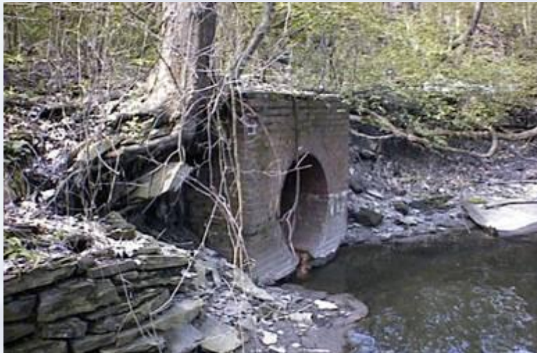
Urban Stormwater Outfall
